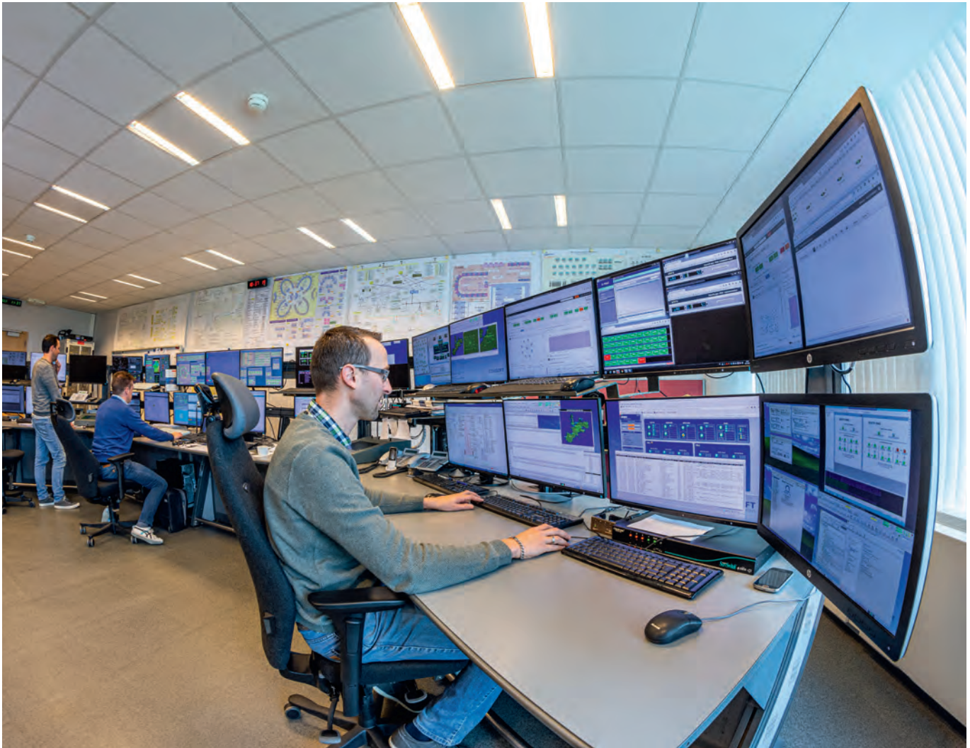
The proper functioning of all CANAC 2 systems is constantly monitored in the Technical Watch Centre (TWC).
