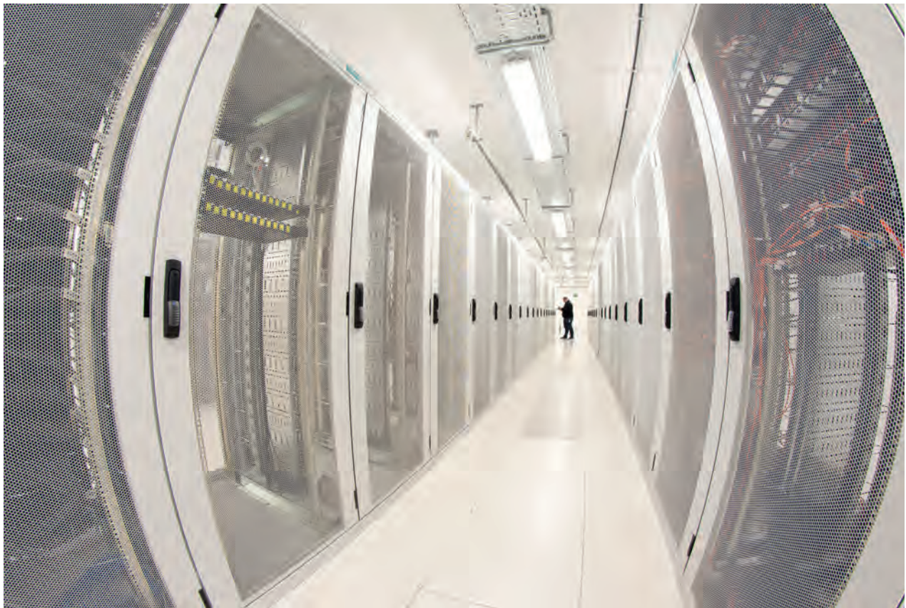
All technical systems are located in two totally redundant rooms situated under the operational room.
