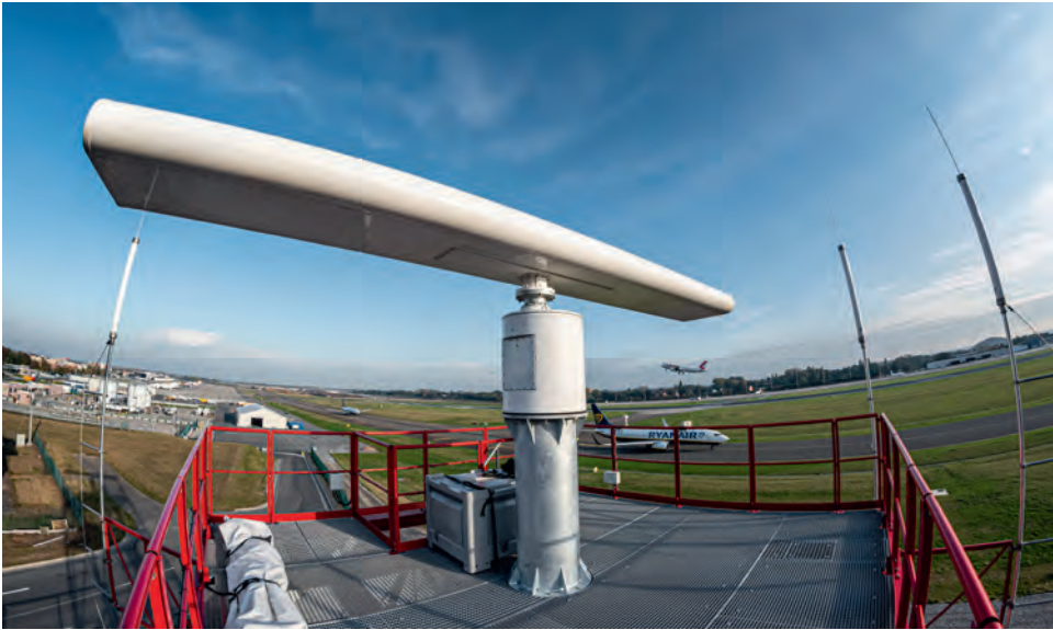
Surface movement radar (SMR) at Brussels South Charleroi Airport
