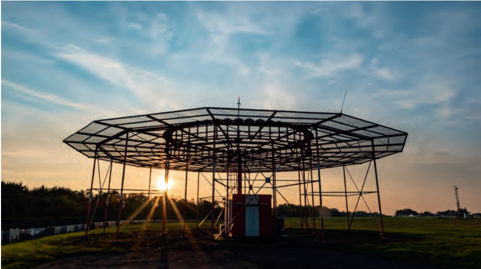
DVOR/DME Navigation ground station at Brussels South Charleroi Airport
